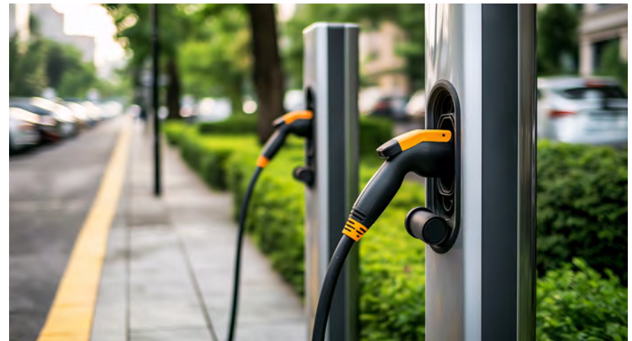
Curbside electric vehicle charging station.
